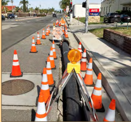
Bypass piping typically set up above the ground as seen here are used to reroute flows out of the sewer pipeline below ground.
