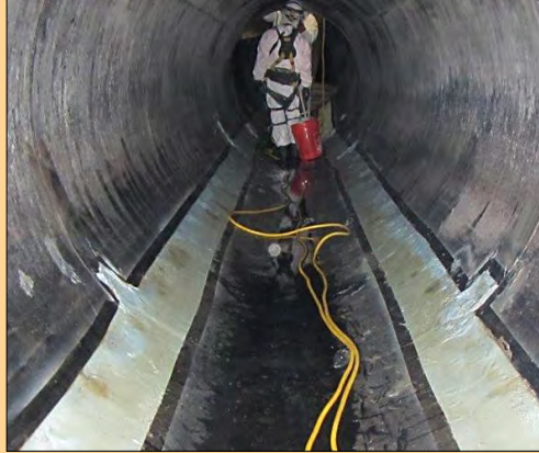
The pipes are large enough for the crews to walk inside of them to make the repairs.
