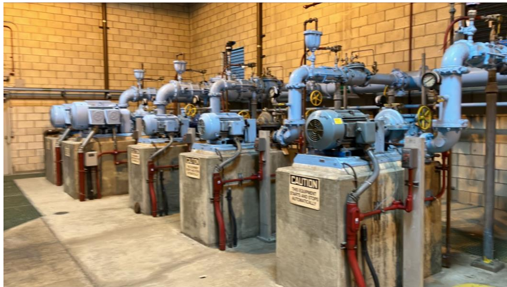
Figure 5 - High Flow and Medium Flow Pumps at Plant No. 2 CWPS
