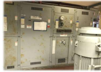
Electrical Equipment at End of Life
