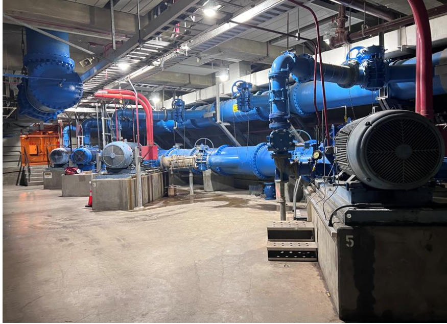
Figure 9 - Pump Room of PWPS
