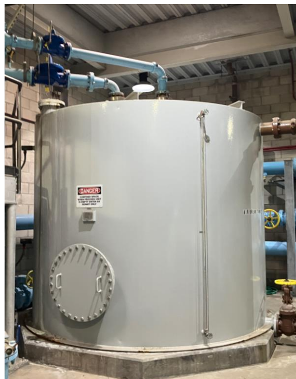
Figure 2 - 6400-Gallon Air Gap Tank Inside the CWPS at Plant No. 1 The second tank (3000-gallon) is not shown.
