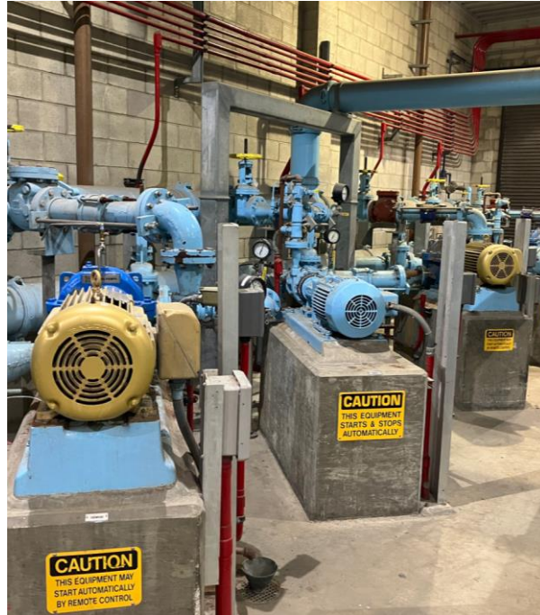
Figure 3 - High Flow and Medium Flow Pumps at Plant No. 1 CWPS
