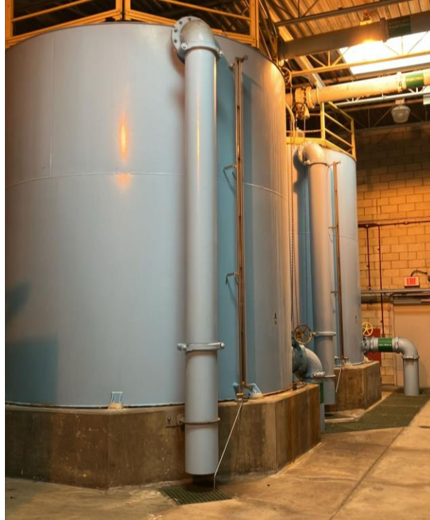
Figure 6 - Two 13,000-Gallon Air Gap Tanks at Plant No. 1 CWPS
