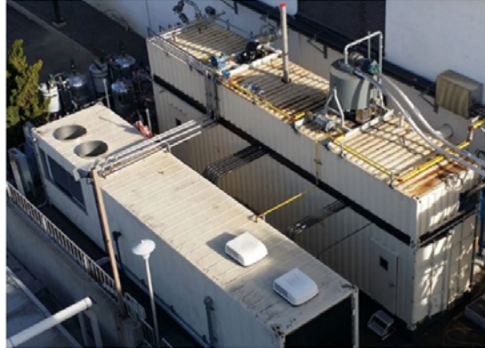
Figure 8: Pyrolysis System at Encina
