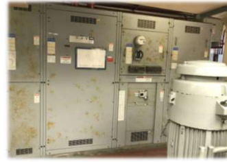
Electrical Equipment at End of Life
