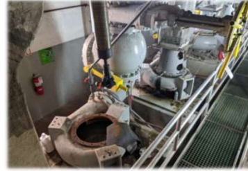
Mechanical Equipment at End of Life
