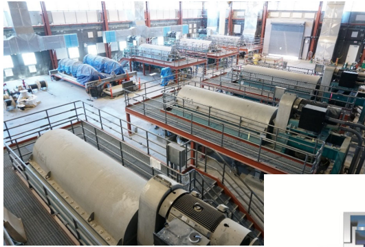
Centrifuge System at Plant No. 1
