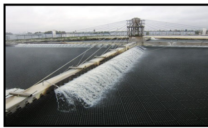
Trickling Filter at Plant No. 1
