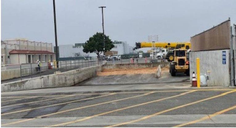
Photo of Plant No. 1 Drying Beds Area
