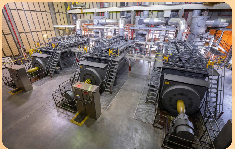
Central Generation facility at Plant No. 1 in Fountain Valley.
