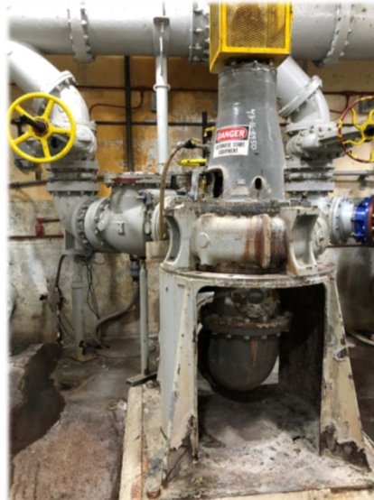
Pump and Structure at End of Life
