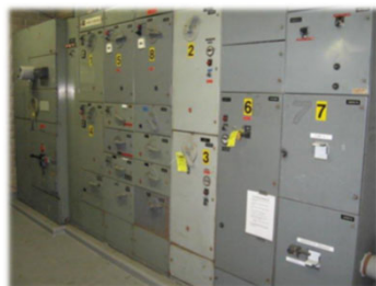
Electrical Equipment at End of Life
