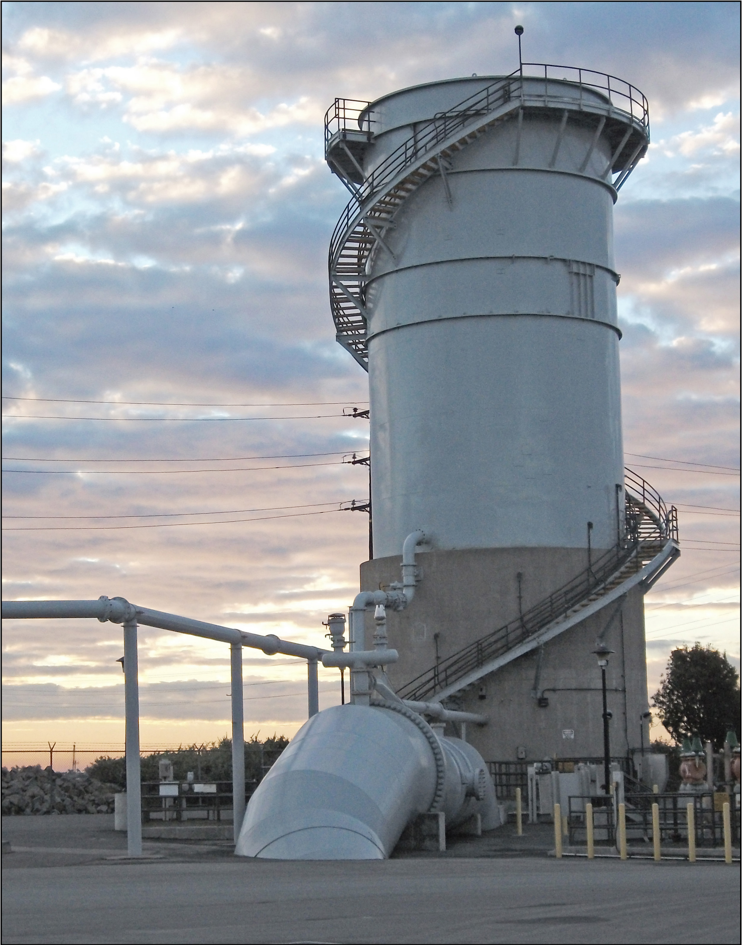
Surge tower at Plant No. 2 in Huntington Beach.
