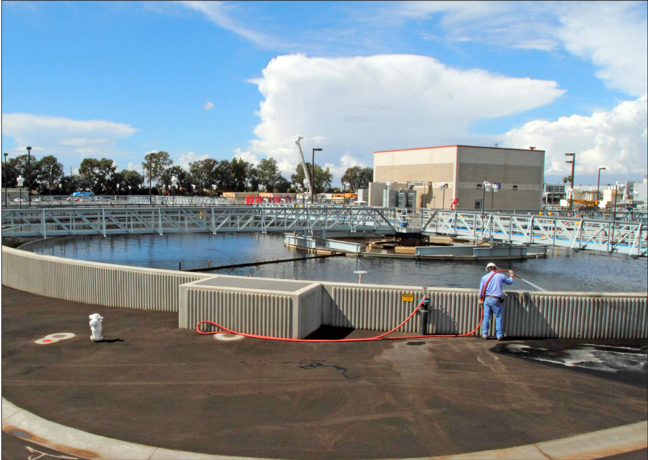
Secondary clarifier at Plant No. 1 in Fountain Valley.
