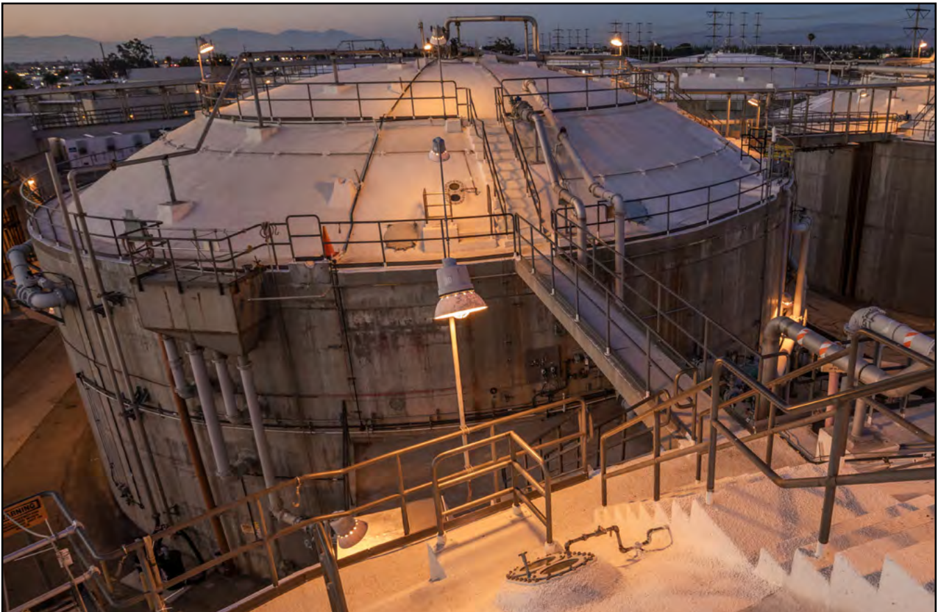
Digesters at Plant No. 1 in Fountain Valley
