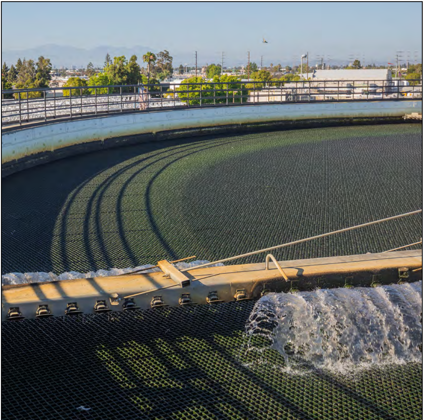
Trickling Filter at Plant No. 1 in Fountain Valley
