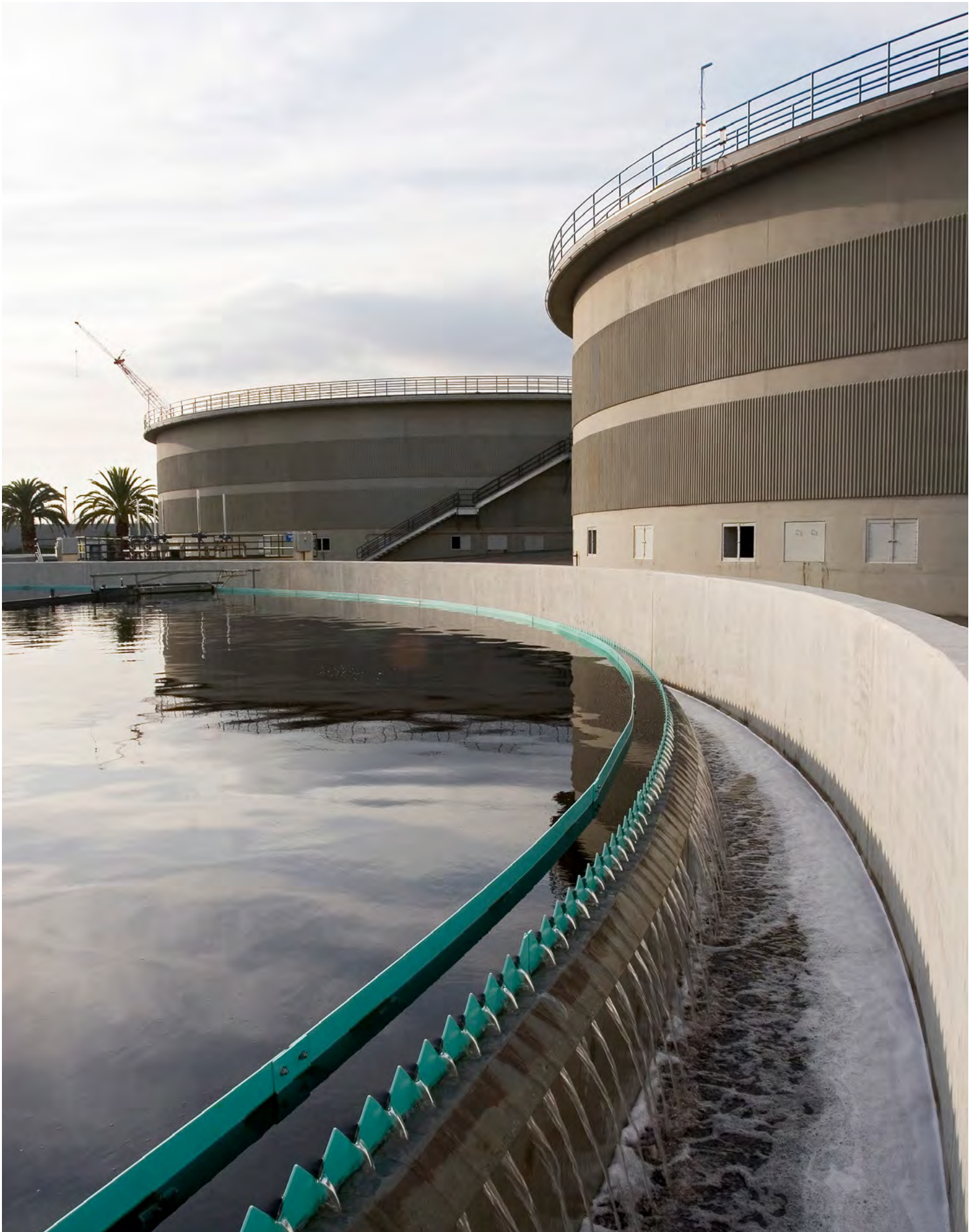
Trickling Filter and Clarifiers at Plant No. 1, in Fountain Valley
