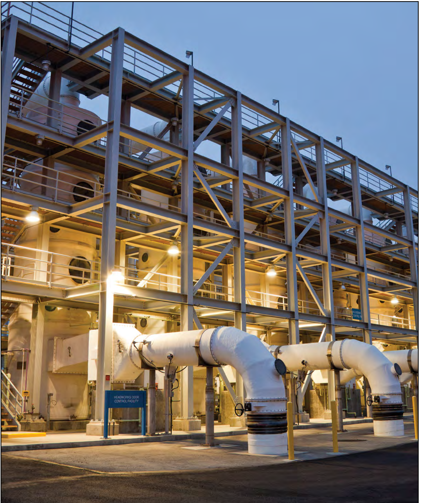
Headworks Order Control Facility at Plant No. 2 in Huntington Beach
