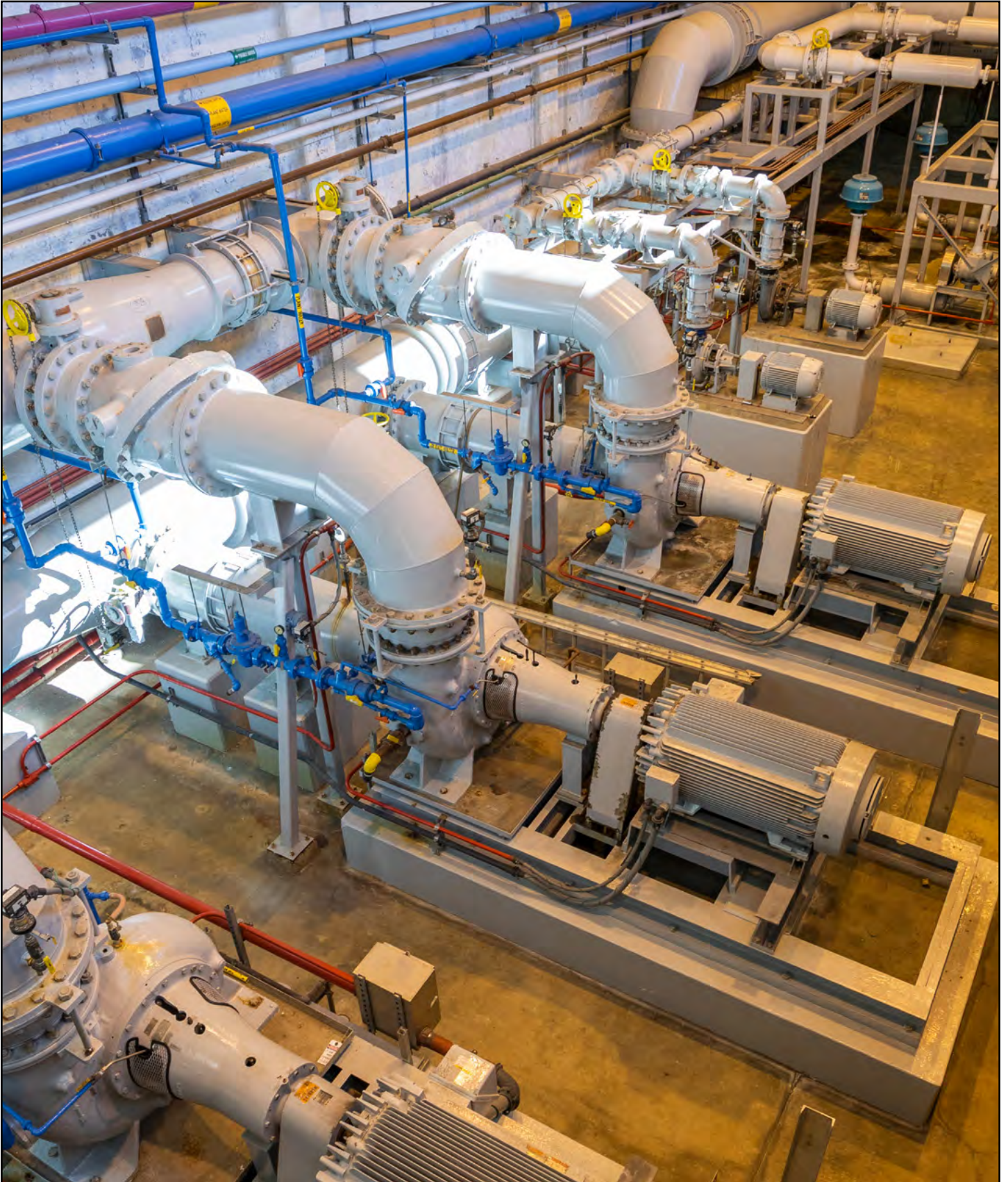
Centrifuge facility at Plant No. 2 in Huntington Beach
