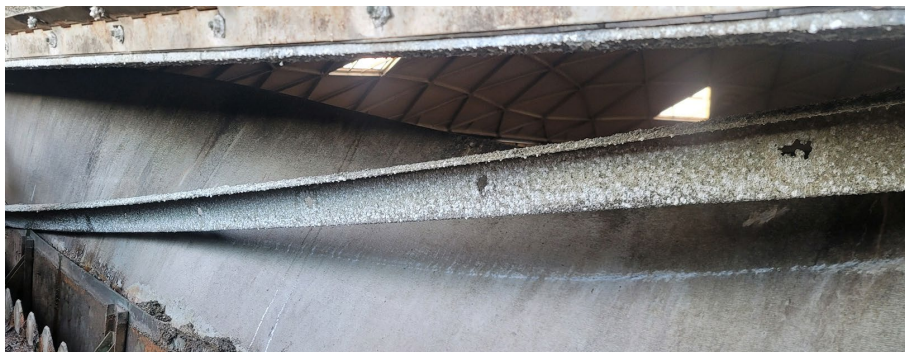
Figure 4: Collapsed baffle wall and aluminum angle
