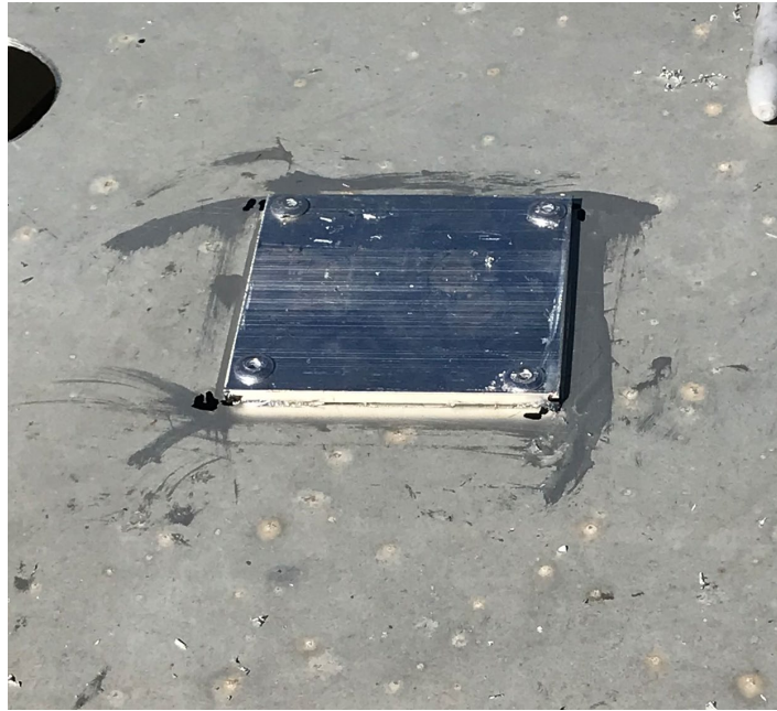
Figure 20: Aluminum patch installed on top of a hole (different basin)
