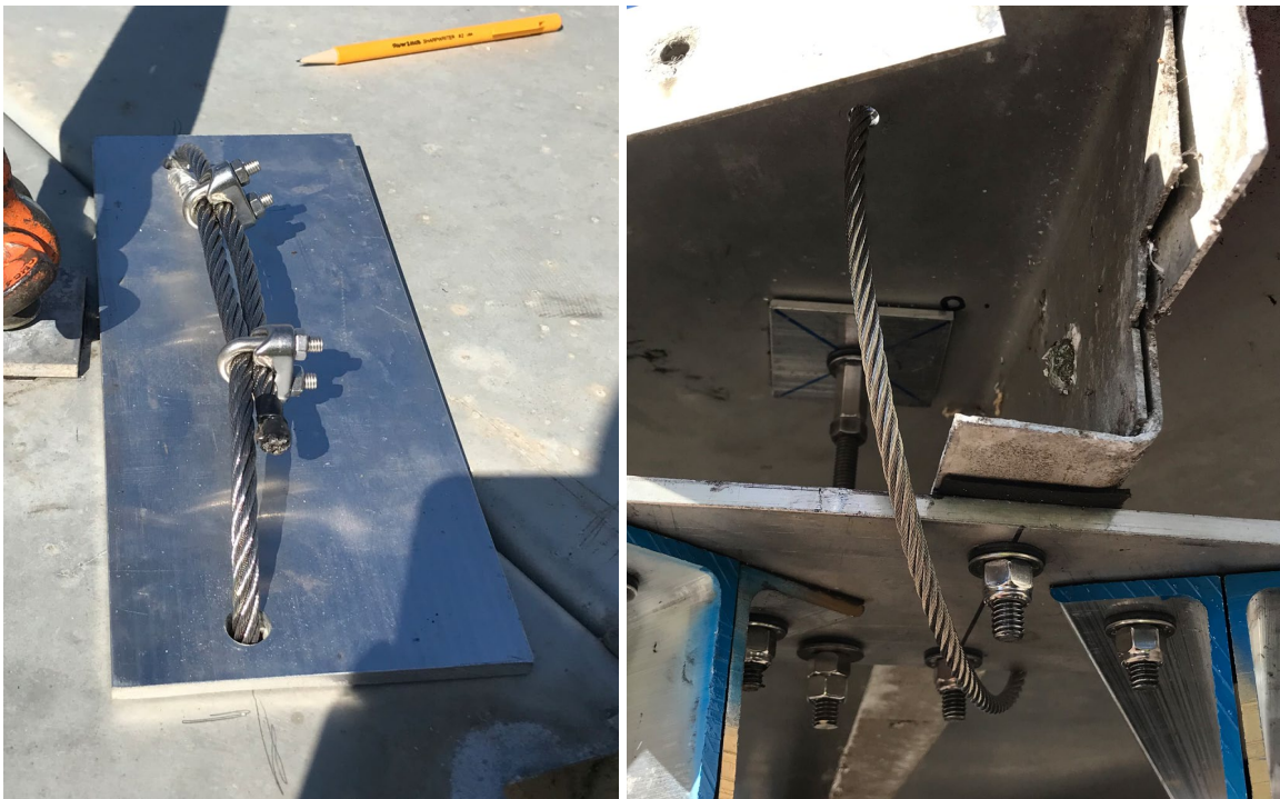
Figure 19: Top and bottom view of installed safety wire (different basin)
