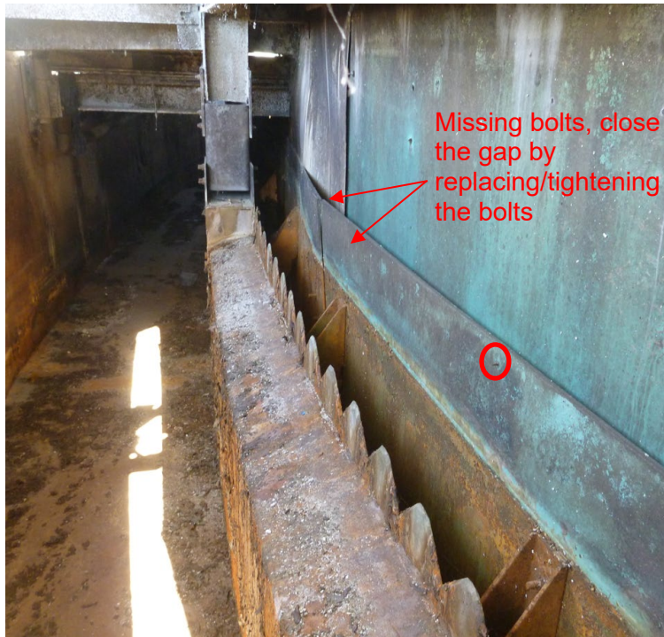
Figure 13: Baffle Wall connection and missing bolts
