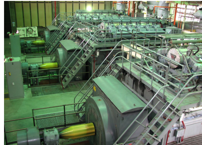
Digester Gas Powered Generators
