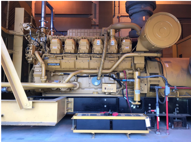
Diesel Powered Backup Generators
