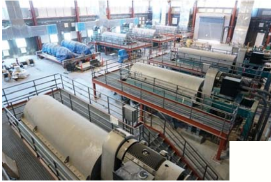
Centrifuge System at Plant No. 1
