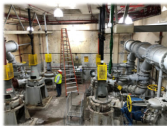
Pump Station Dry Well
