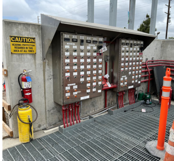
Sunflower Pump Station Control Panels
