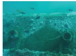
End Structure Flap Gate Hinges
