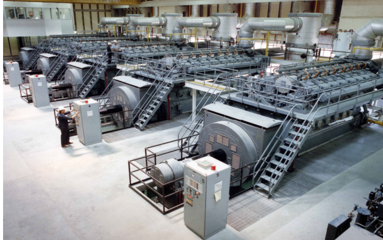
Plant No. 2 Central Generation Engines
