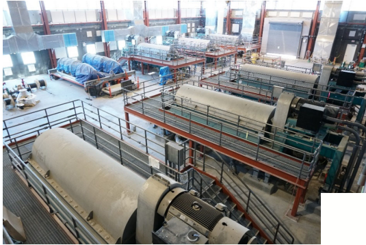
Centrifuge System at Plant No. 1
