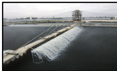
Trickling Filter at Plant No. 1
