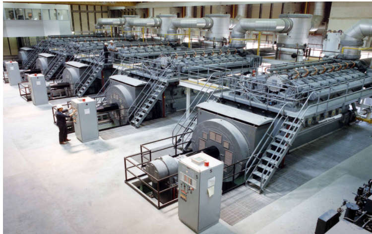
Plant No. 2 Central Generation Engines
