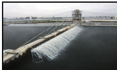
Trickling Filter at Plant No. 1
