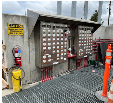
Sunflower Pump Station Control Panels
