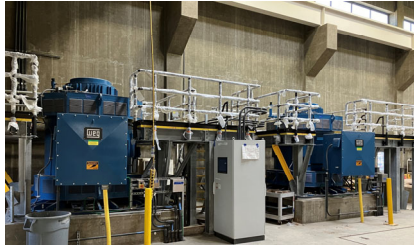
OOBS Pumps (2,650 HP)
