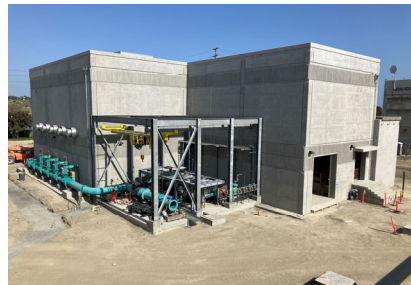
Low Flow and Plant Water Pump Stations
