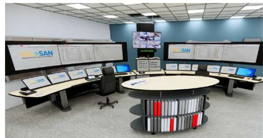
J-120A Control Room Reconfiguration
