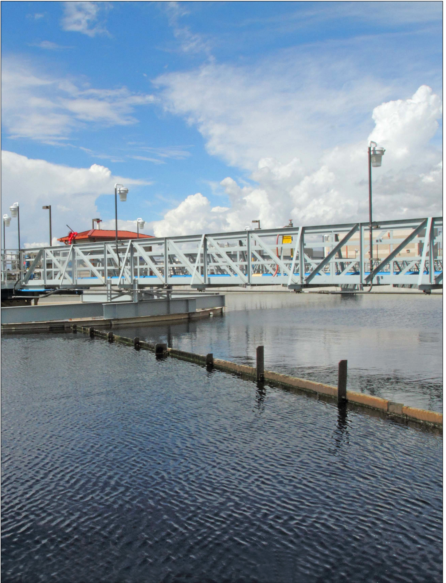
Secondary Clarifier Plant No. 1 in Fountain Valley.
