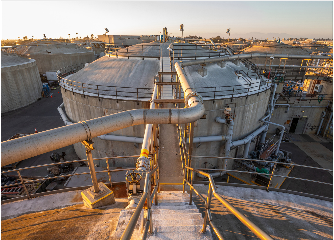
Digesters at Plant No. 2 in Huntington Beach.
