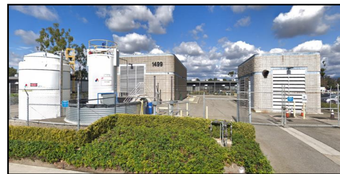
Main Street Pump Station
