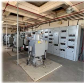
Return Activated Sludge Pump Station Electrical
