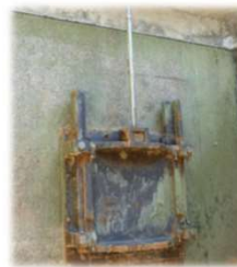
Corroded Slide Gates – Difficult to Open/Close
