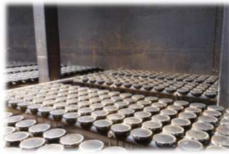
Worn/Damaged Diffusers – Impacts Energy Consumption and Performance
