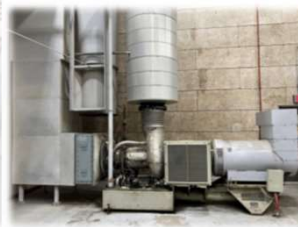
Standby Power Turbine Generator
