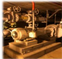
Waste Activated Sludge Pumps
