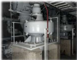
Return Activated Sludge Pumps
