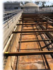
Worn Sludge Collectors
