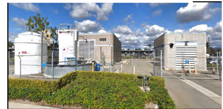
Main Street Pump Station
