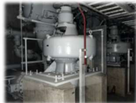
Return Activated Sludge Pumps
