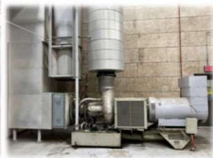
Standby Power Turbine Generator
