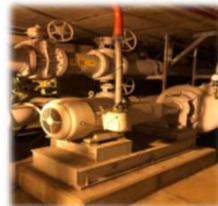
Waste Activated Sludge Pumps
