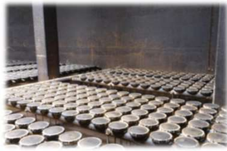
Worn/Damaged Diffusers – Impacts Energy Consumption and Performance
