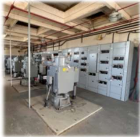
Return Activated Sludge Pump Station Electrical
