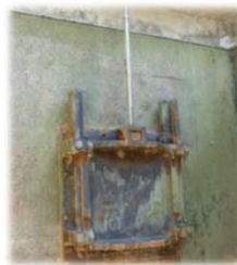
Corroded Slide Gates – Difficult to Open/Close
