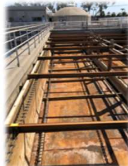
Worn Sludge Collectors
