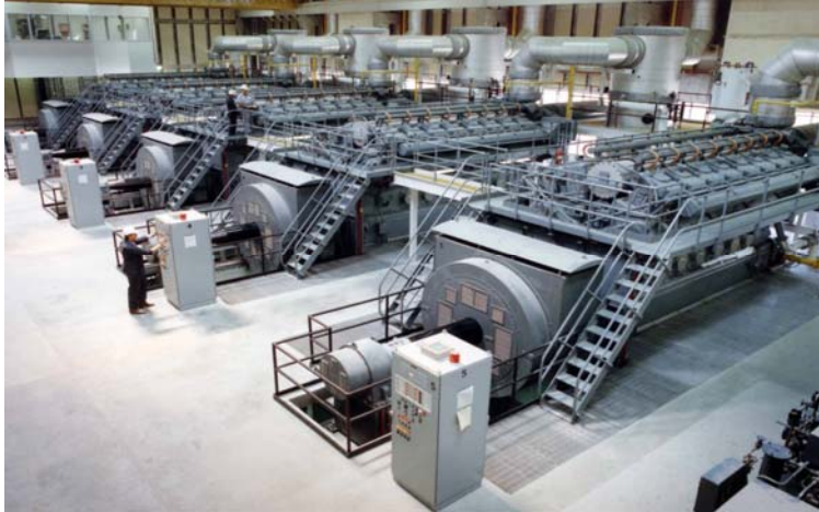
Plant No. 2 Central Generation Engines
