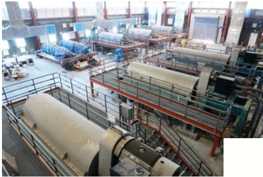
Centrifuge System at Plant No. 1
