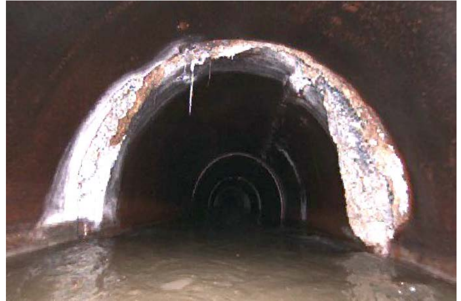
Calcium deposit at pipe joint
