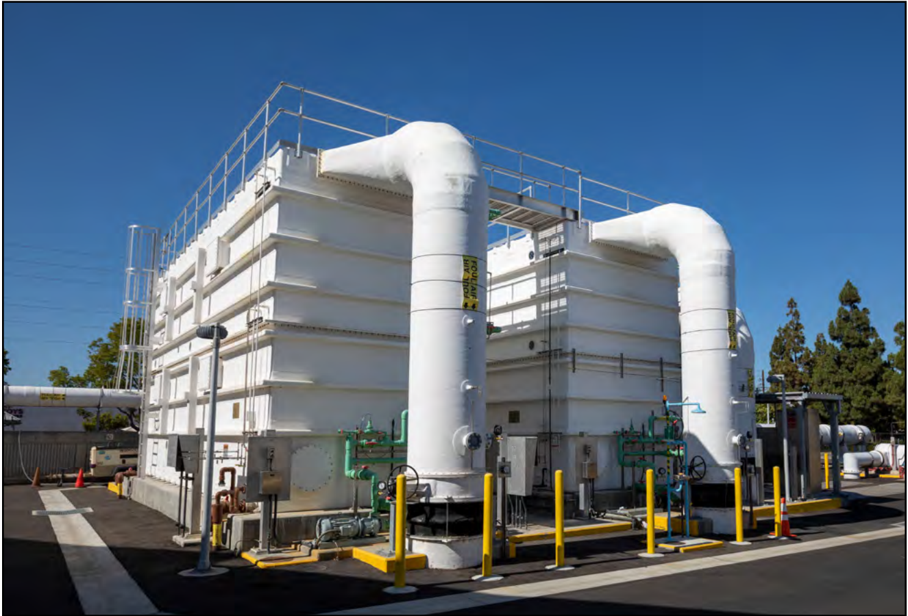
Odor Control Air Scrubbers at Plant No. 1 in Fountain Valley
