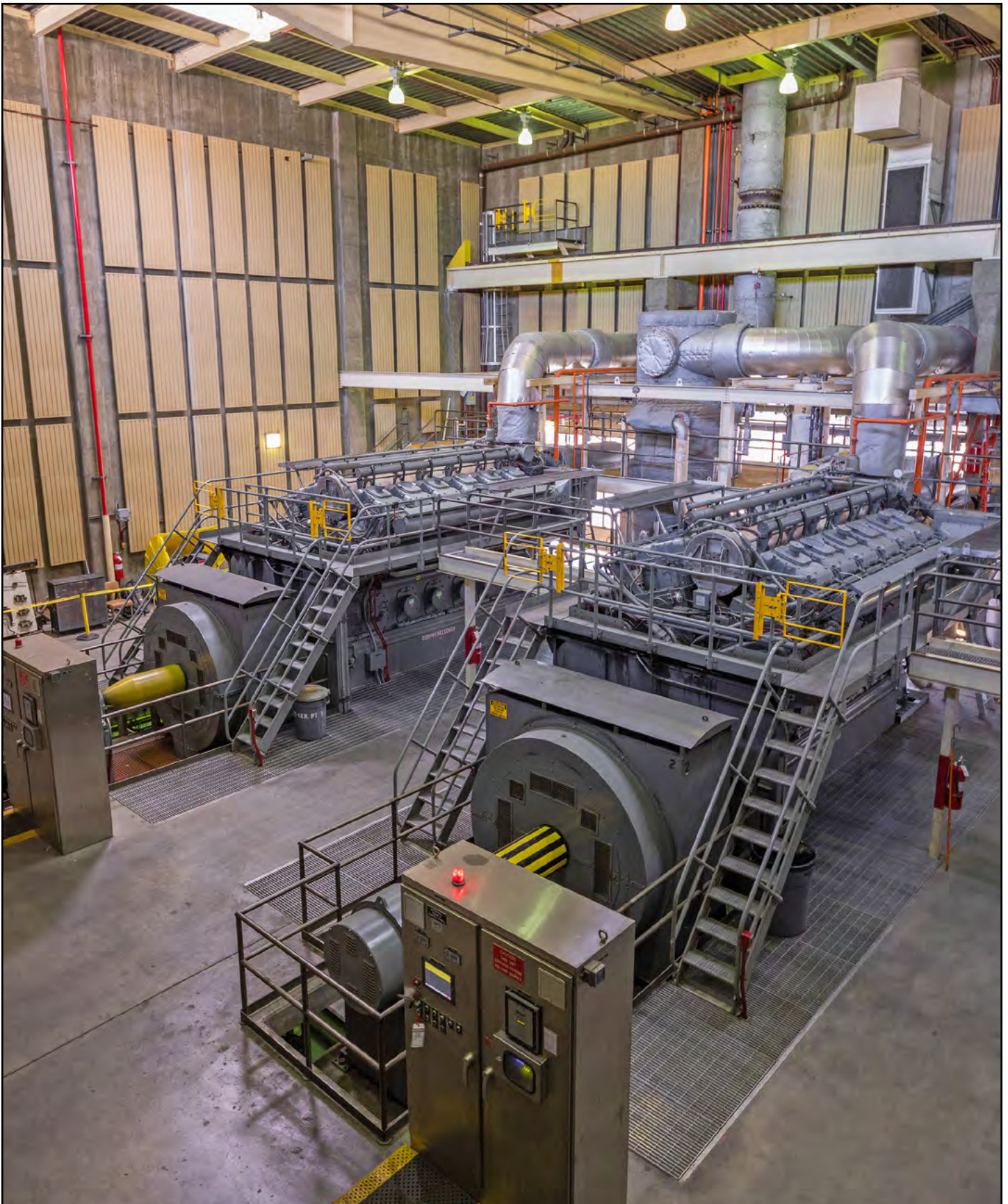
Central Generation engines at Plant No. 1 in Fountain Valley
