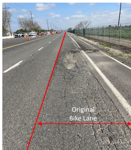
Damage after Construction
