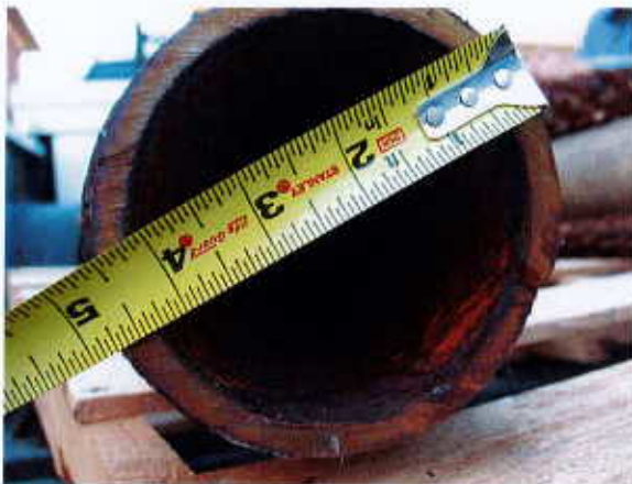
Corrosion is evident in this wastewater pipe from Los Angeles County. (Image: Los Angeles County Public Works Department)
