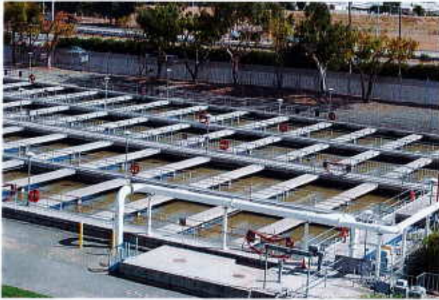
Part of a wastewater treatment plant in Contra Costa County. (Image: File)
