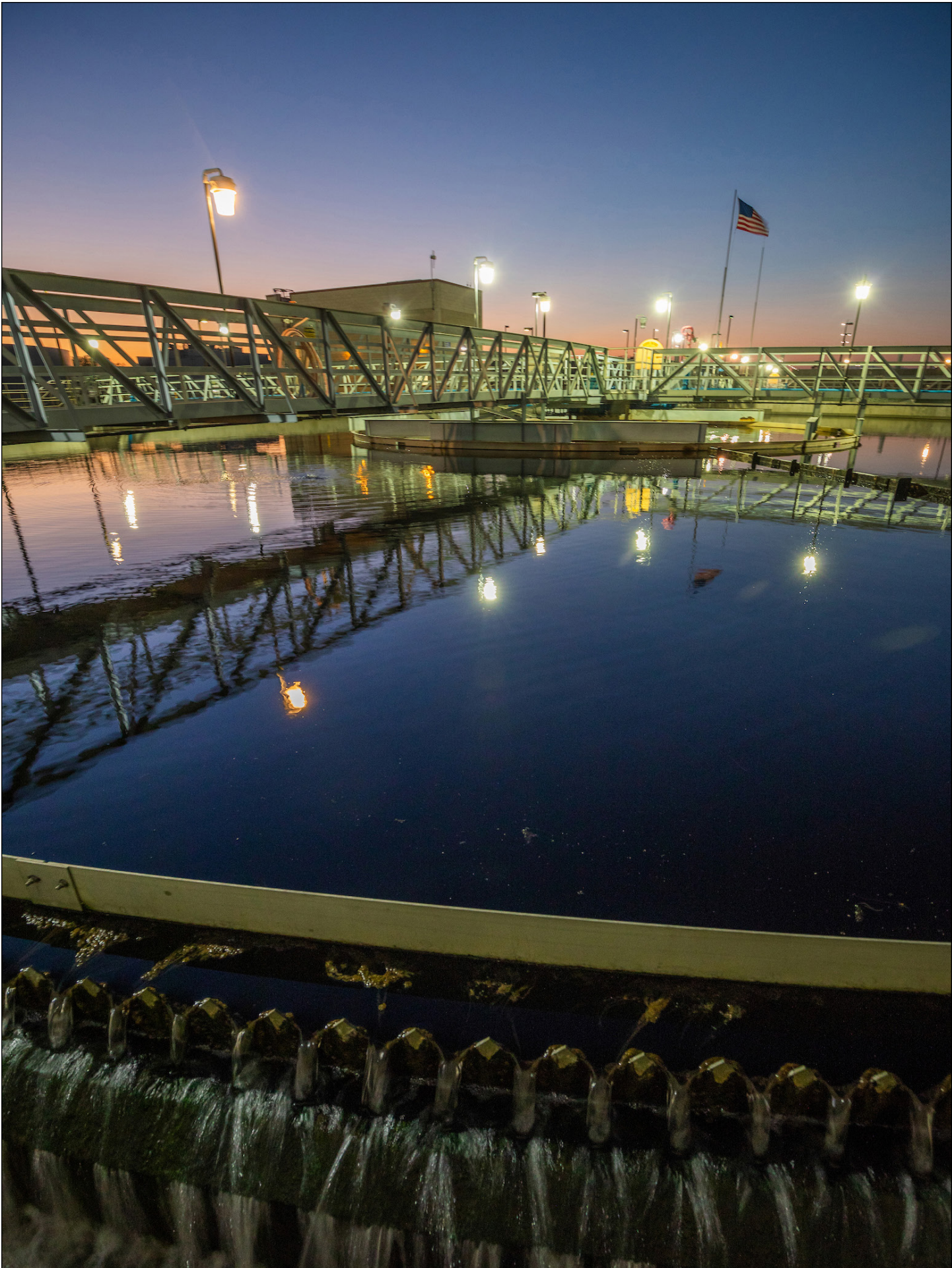
Secondary clarifier at Plant No. 1 in Fountain Valley.
