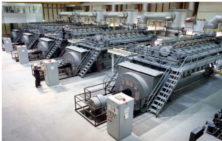
Plant No. 2 Central Generation Engines
