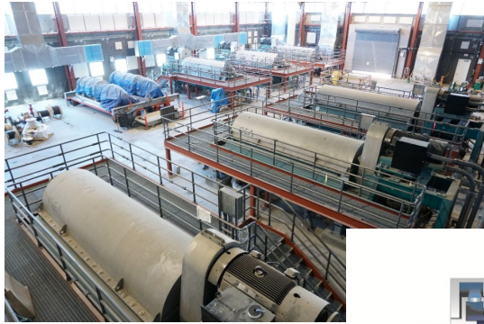
Centrifuge System at Plant No. 1
