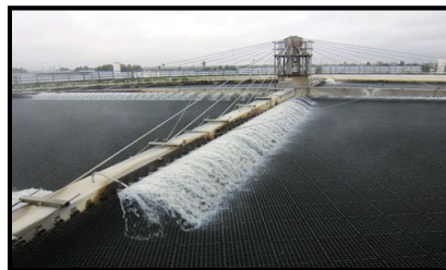
Trickling Filter at Plant No. 1
