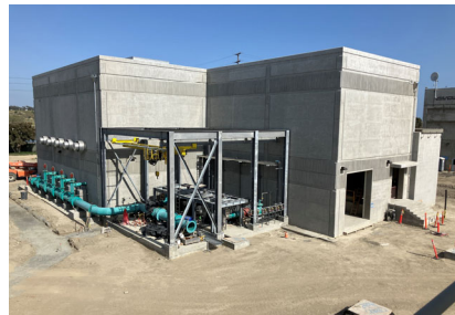
Low Flow and Plant Water Pump Stations
