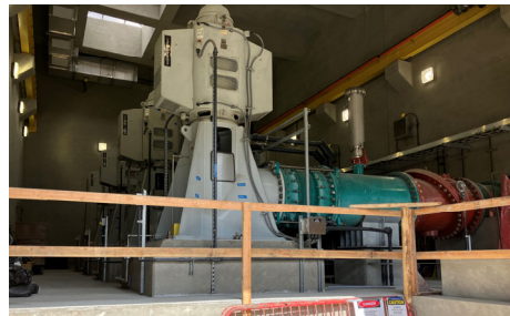
Low Flow Pumps
