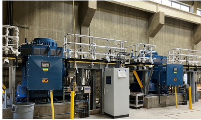
OOBS Pumps (2,650 HP)
