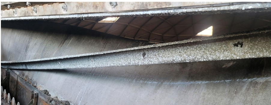
Figure 4: Collapsed baffle wall and aluminum angle
