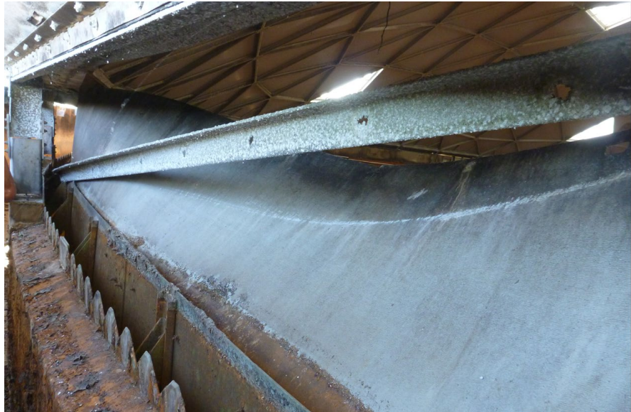
Figure 12: Collapsed baffle wall in basin G
