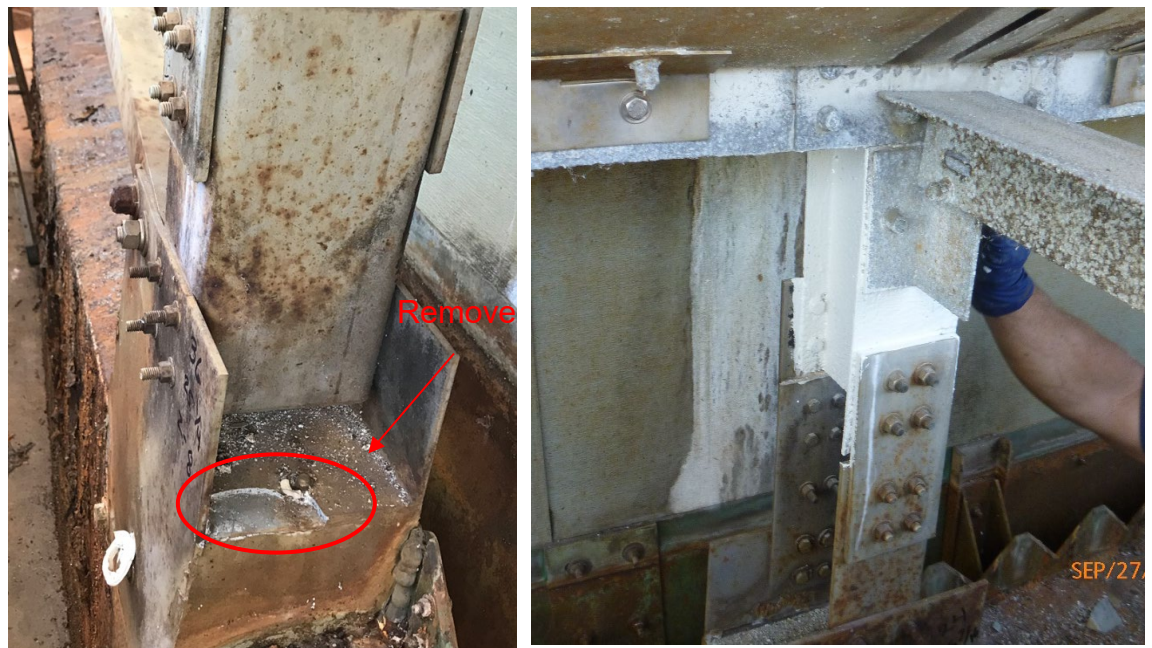
Figure 5: Partially removed mortar liner above a steel plate (different basin)
