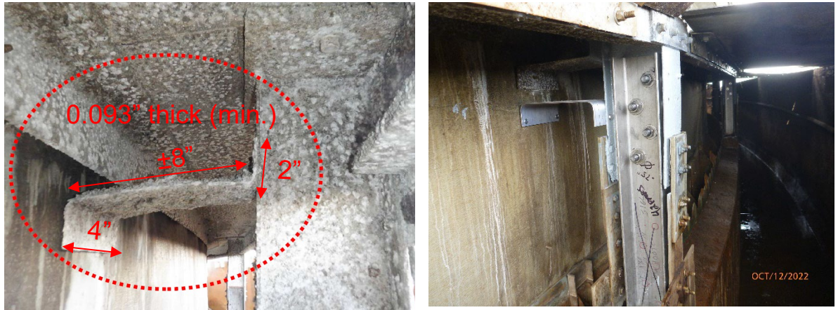
Figure 10: Aluminum angle and "Z" clip providing support to the baffle wall (Typical)
