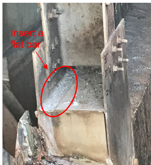
Figure 6: Exposed steel plate (different basin)
