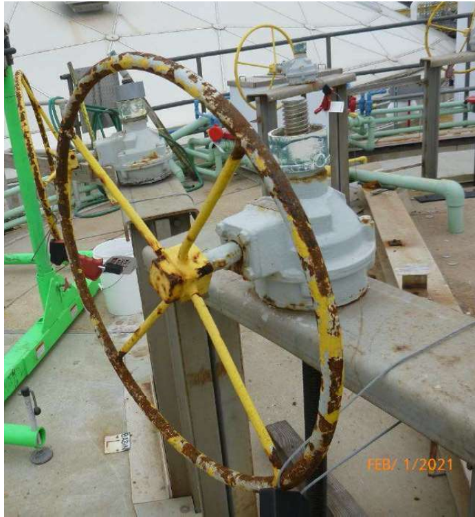
Picture 4: Corroded handwheel and bevel gear operator
