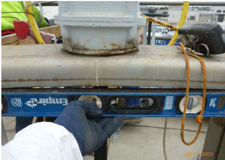
Picture 5: Bent gate top frame
