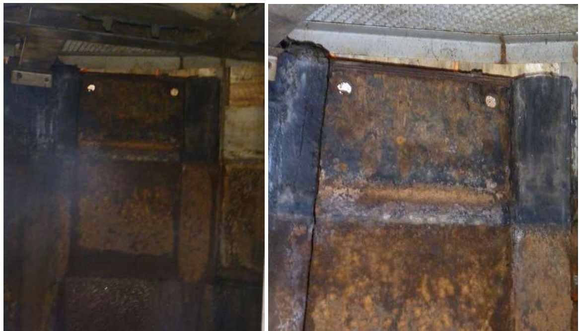
Picture 8: Corroded carbon steel bulkhead from center of distribution structure
