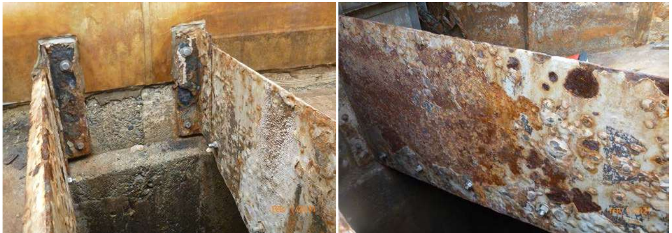
Picture 12: Corroded steel weir plates
