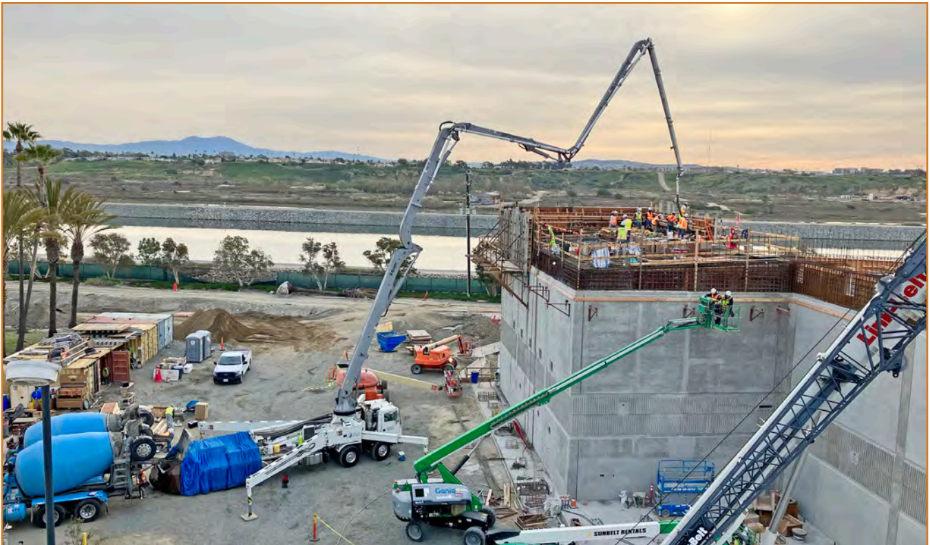
New Low Flow Pump Station at Plant No. 2 that pumps to our ocean outfall.
