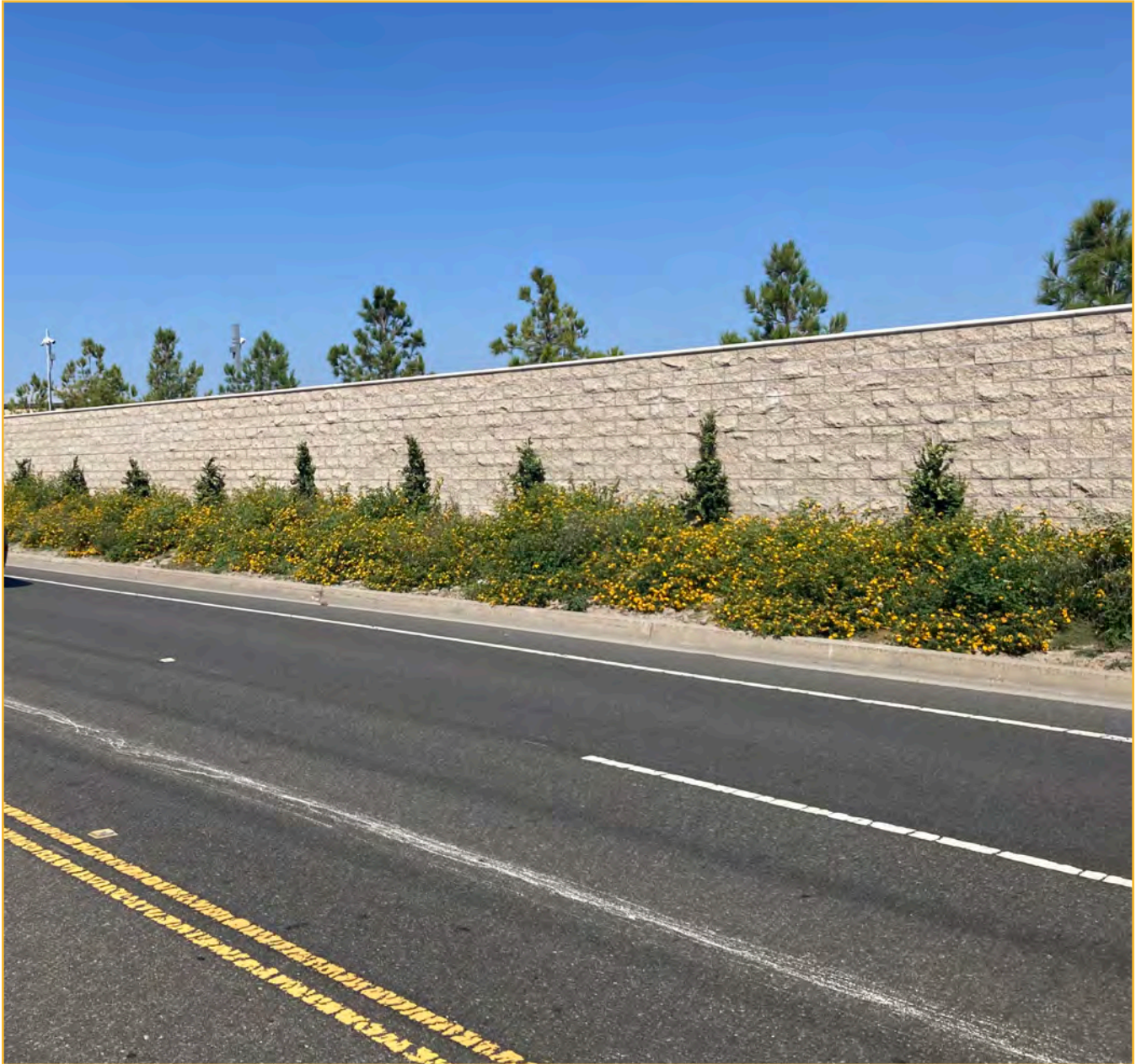
Street view of the new wall and landscaping for the Southern Perimeter Security and Utility Improvements Project.
