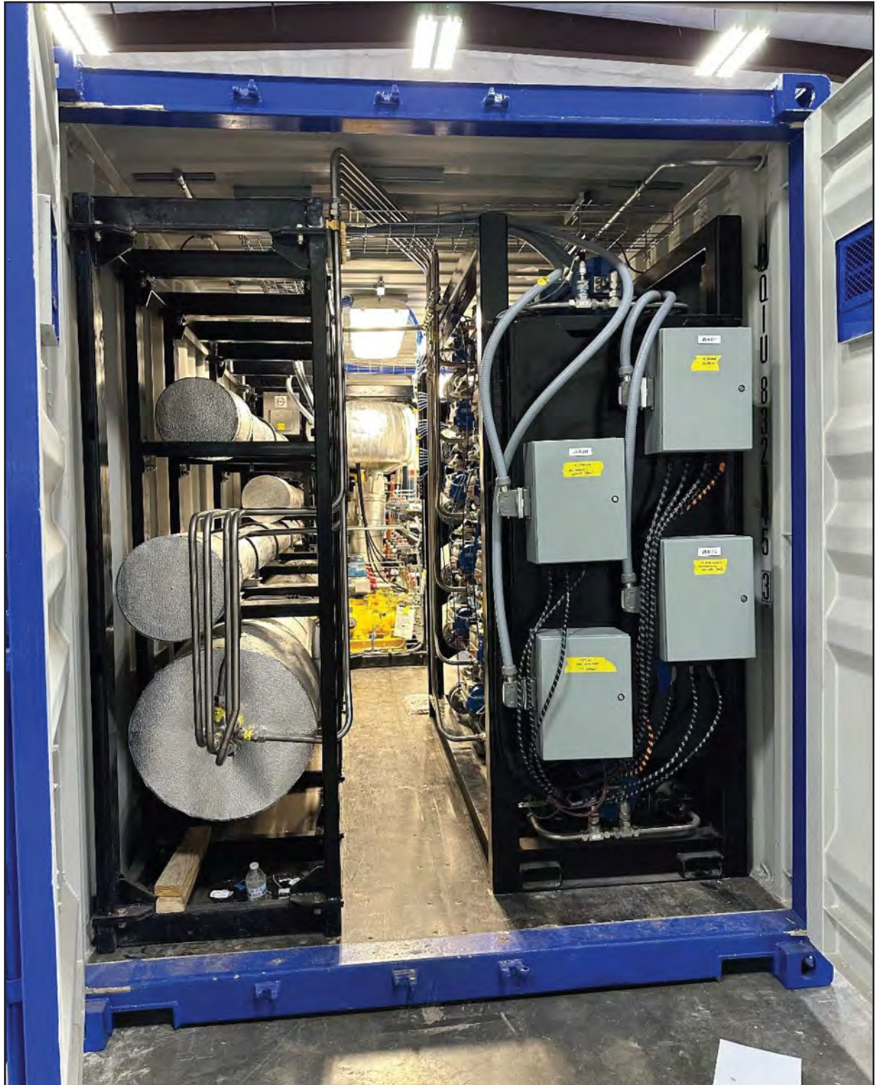
Heat exchanger skid and slurry pump skid fully installed into AirSCWO system.
