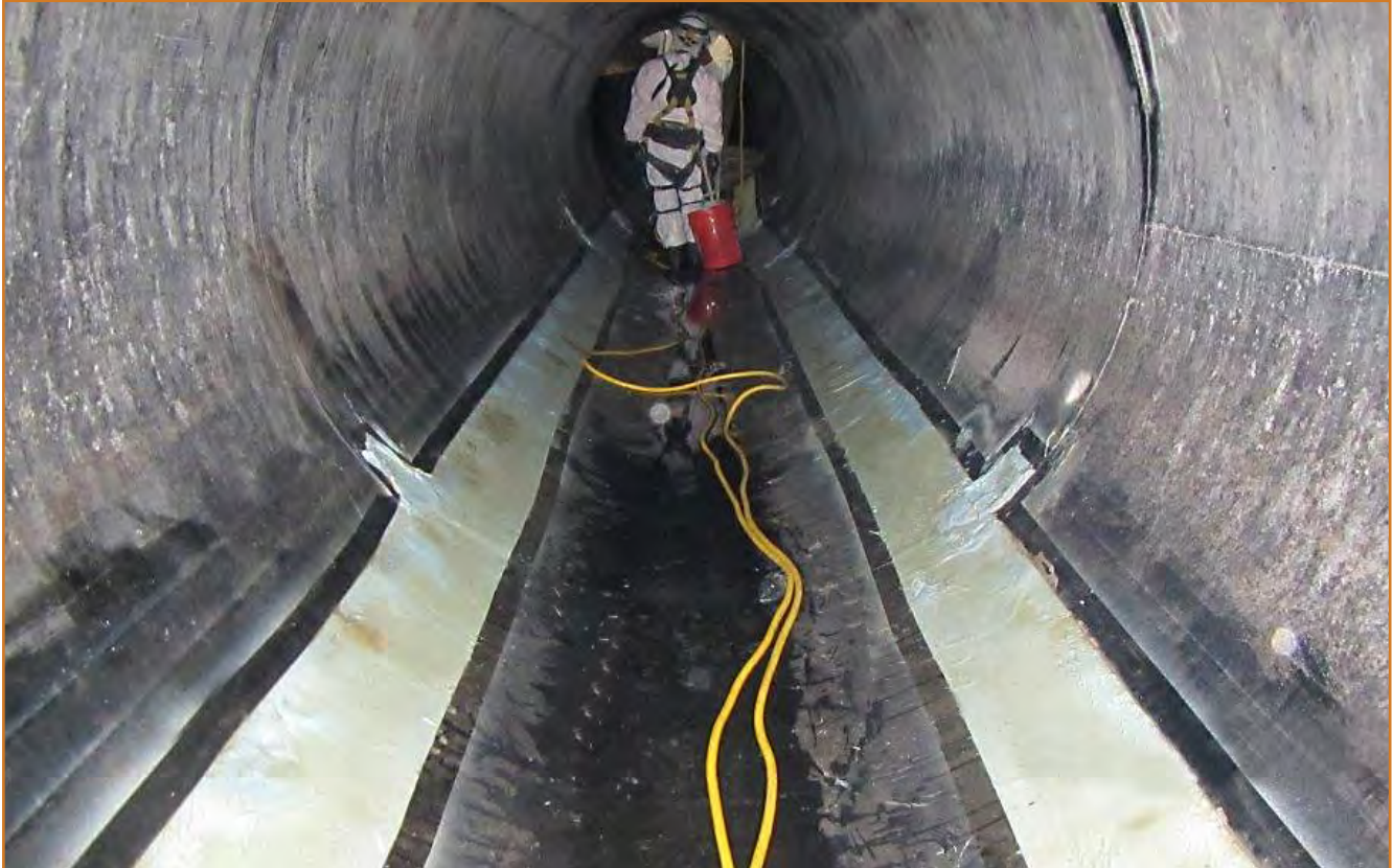
Crews working inside the pipeline on the Sunflower and Red Hill Interceptor Repair Project.
