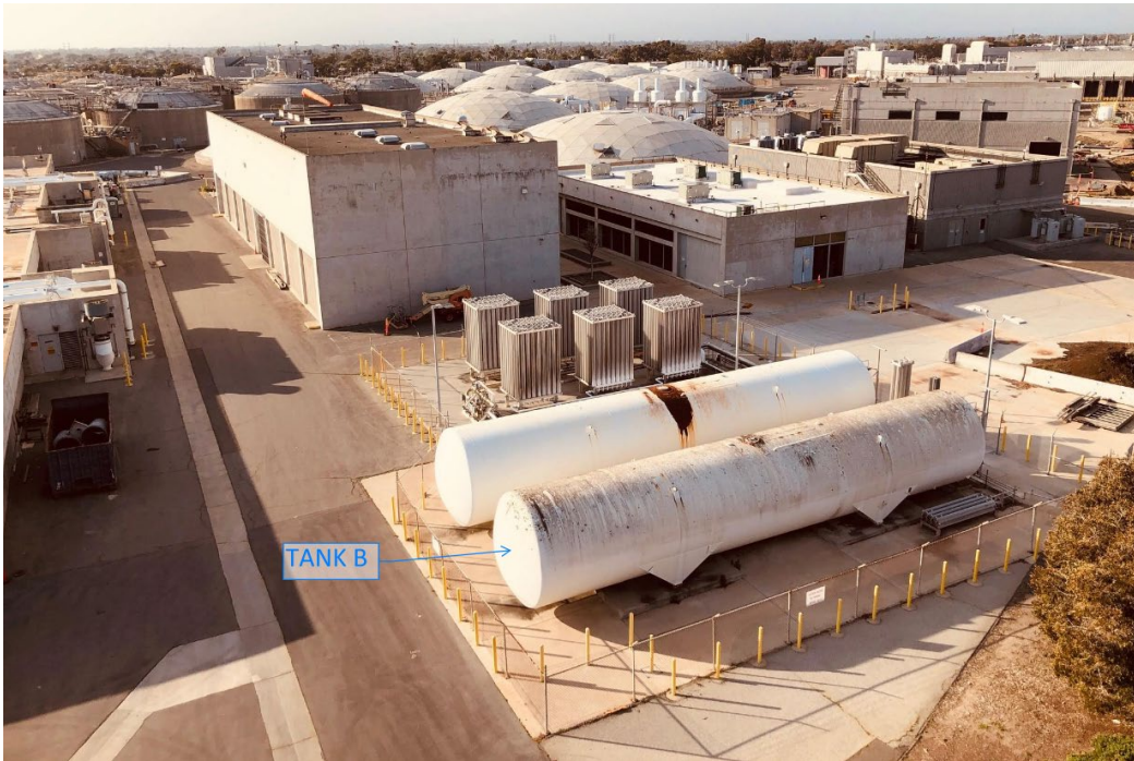
Figure 2: Tank B instrumentation.
