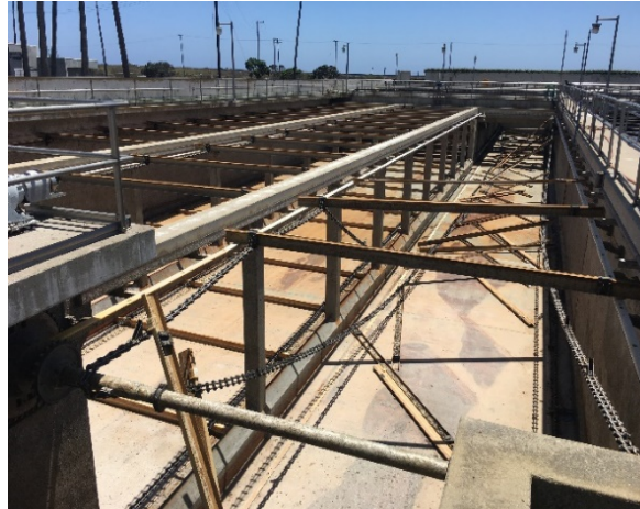
Broken Clarifier Mechanism
