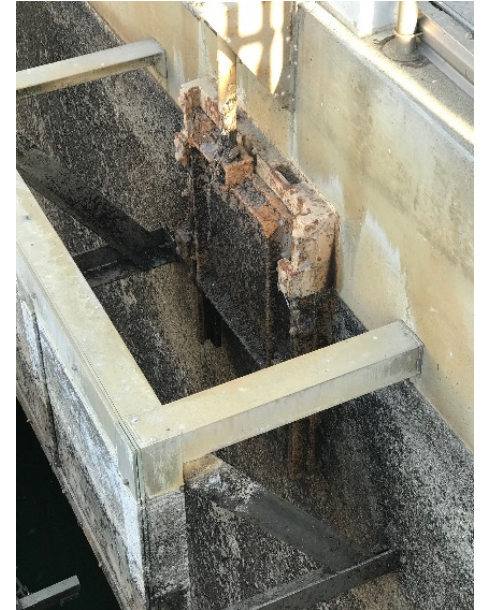
Corroded/Broken Inlet Gates
