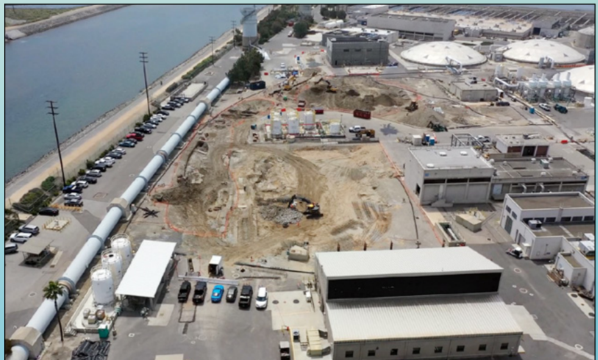
Four new Primary Clarifiers will be constructed at Plant No. 2 in Huntington Beach.
