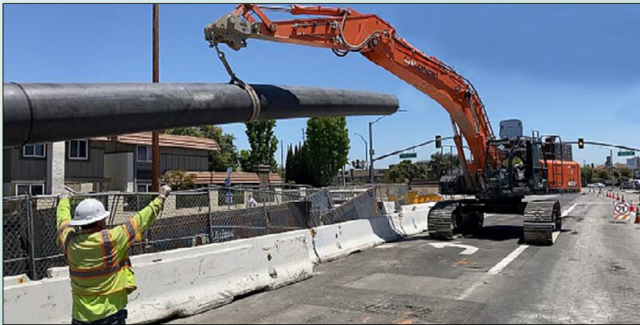
LEFT: Segments of HDPE pipe are fused together. Fun fact: Each 50-foot segment of HDPE pipe weighs 5,000 lbs.
